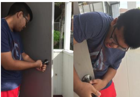
Thank you Gavin Nishihira for installing the new doorknob on the side of the church! It's much easier to open and lock!
